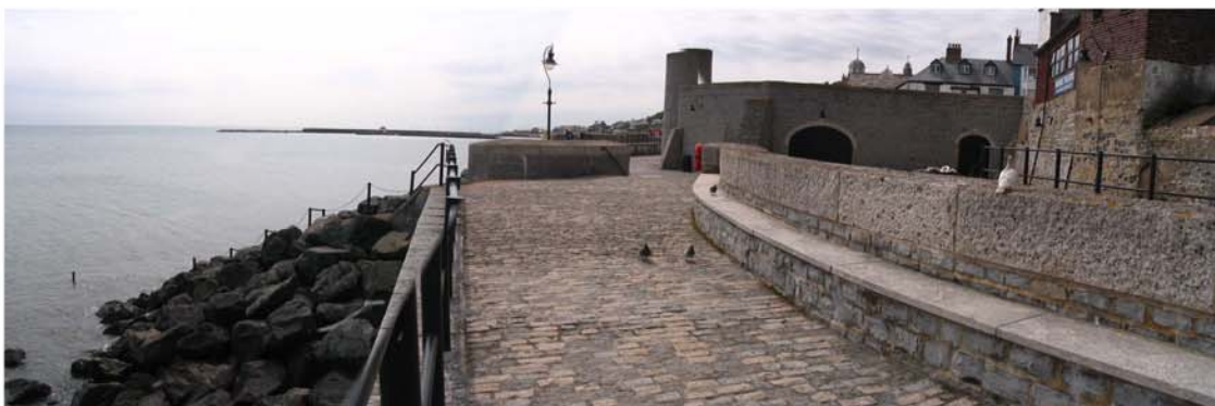
A cross section of the sea defences at the Marine Theatre site. Image copyright RGS-IBG.
