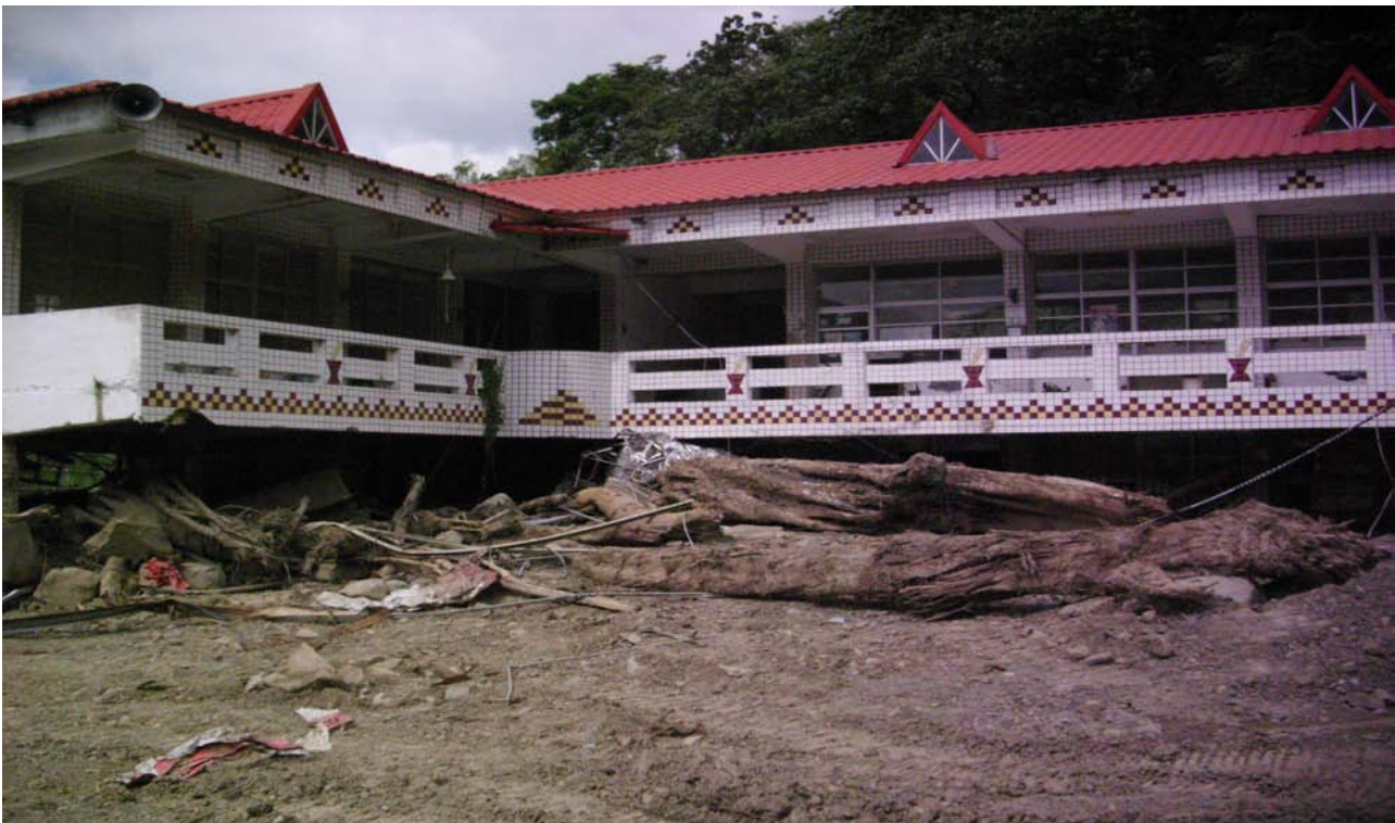
Fig. 48. Nangisalu Elementary School. Evacuation Centre for Namisalu village during Typhoon Morakot. For those participants who did not leave their houses responses indicated that participants were reluctant to leave their homes and/or didn't think the storm would be so heavy. In one instance the participant stated that he was not told about evacuation procedures (it can be concluded that the
