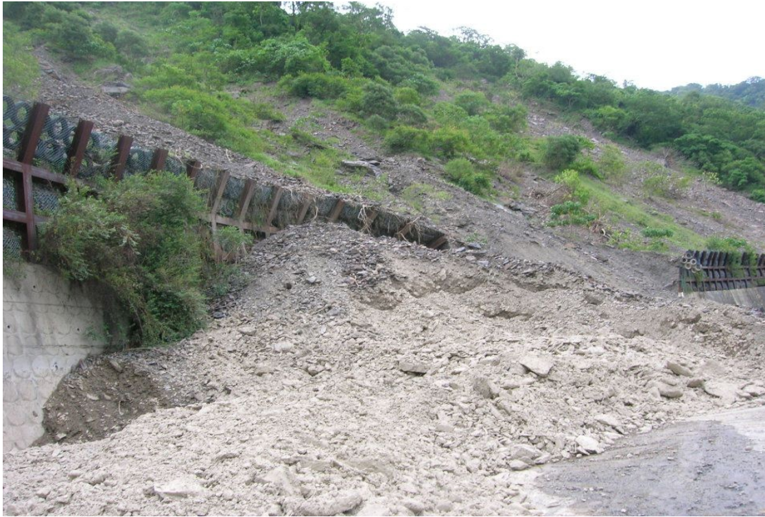
Fig. 15. Maolin entrance landslide
